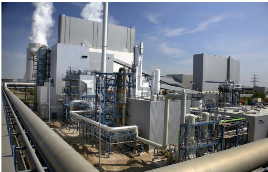
Boiler assembly at Vattenfall's Schwarze Pumpe pilot CCS plant. For more on the Schwarze Pumpe project, turn to page 15
